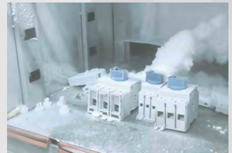
High Low-Temperature Humid-Heat Test
